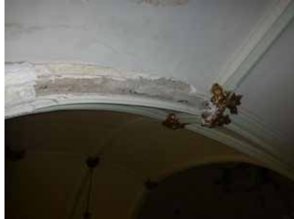
61. Deterioration of the ceiling (ERA, 2015).
