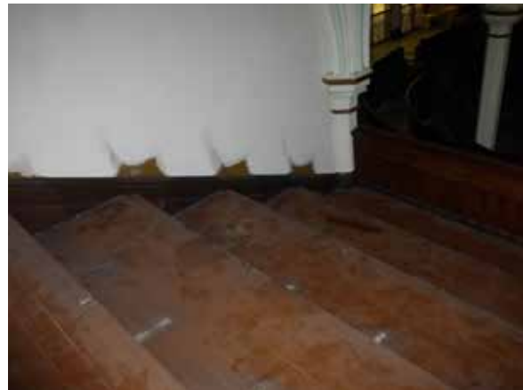
63. Missing pews in the gallery (ERA, 2015).
