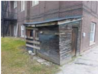
42. Wooden shed on the west facade of the building, to the south (ERA, 2015).
