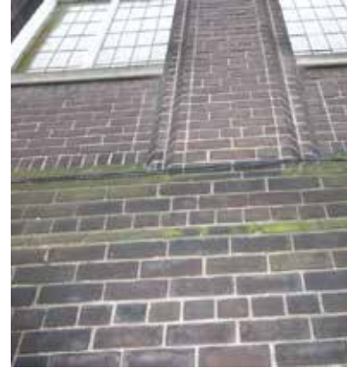
44. Organic growth on the Sunday School addition (ERA, 2015).
