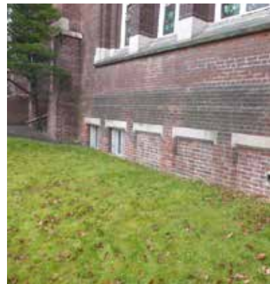
46. Bricked in windows along the north elevation of the church building (ERA, 2015).
