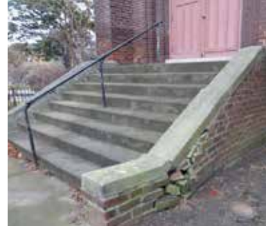
48. Entrance stair deterioration (ERA, 2015).
